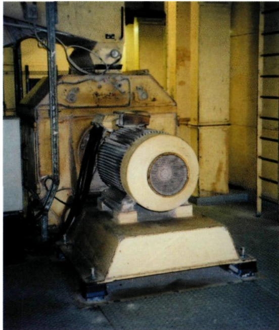
Figure 15 Anti-vibration mounts isolate a grinder from the supporting surface
