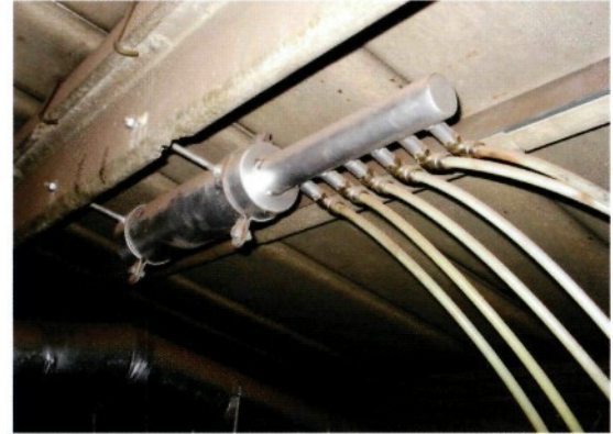
Figure 21 Multiple air exhausts piped to a manifold and silencer
